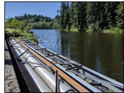
Exhibit 3.47 Utilities line routed along Deschutes Parkway. View from parkway of Percival Cove
