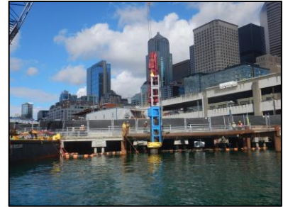
Exhibit 2.12 Pile driver along Seattle's waterfront (Source: Washington State Department of Transportation https://creativecommons.org/licenses/by-nc-nd/2.0/ )
