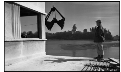
Exhibit 3.52 Deschutes Dam construction, April 8, 1950 (Source: The Susan Parish Collection of Photography, Washington State Archives)
