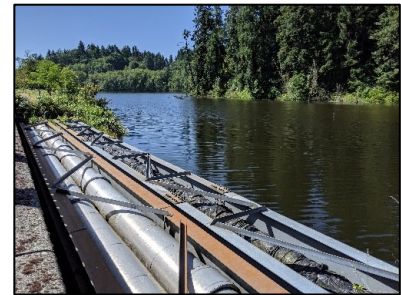
Exhibit 3.68 Utilities line routed along Deschutes Parkway. View from parkway of Percival Cove
